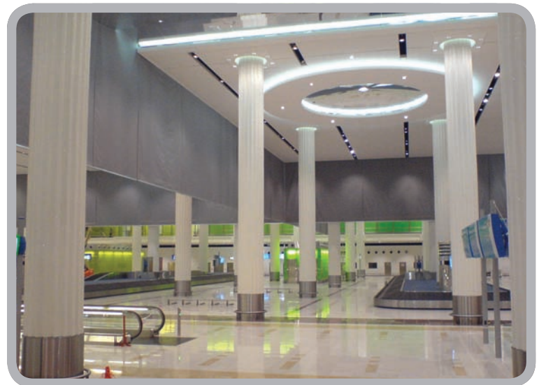
Dubai International Airport, UAE - Reservoir Smoke Curtains
